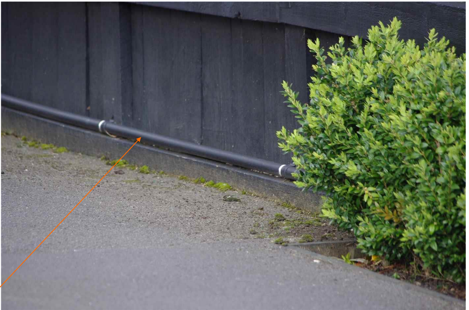
Narrow pipe along bottom of fence in similar colour. Visual impact minimal.
